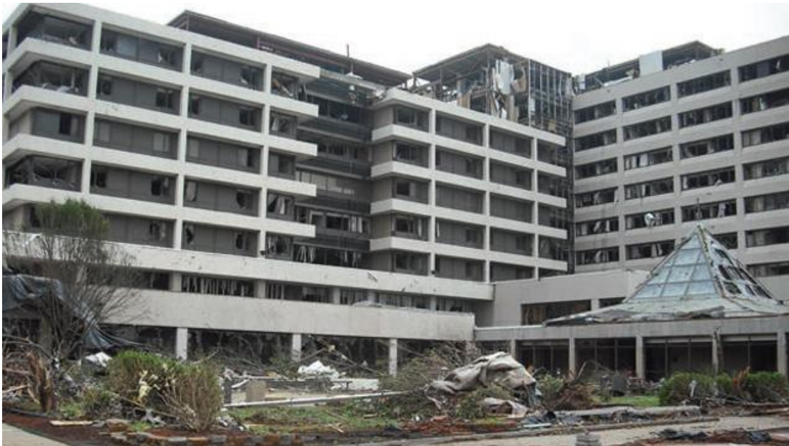
Figure 4: Damage to St. John's Regional Medical Center in Joplin, Missouri following the 2011 tornado [19]
